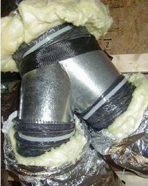
INCORRECT: No Sealant
