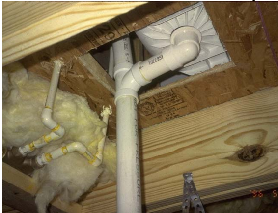
INCORRECT: Drain Penetration Open
