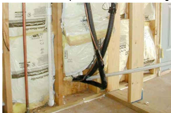
INCORRECT: Compression and Poor Coverage
