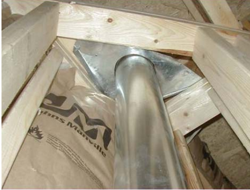
INCORRECT: Improperly Capped Chase
