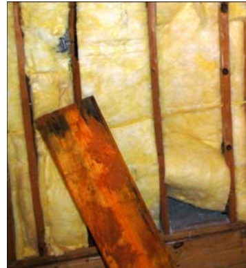
INCORRECT: Unfilled Cavity
