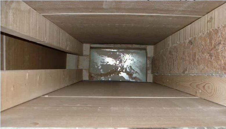
INCORRECT: Unlined Cavity as Supply
