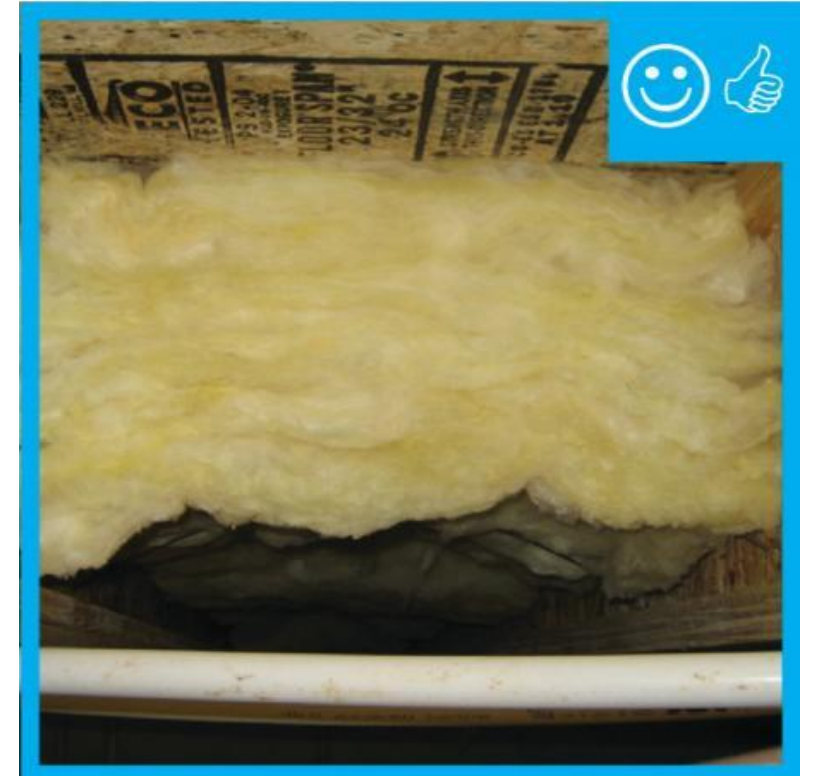
Sub-floor insulation is properly installed and supported
