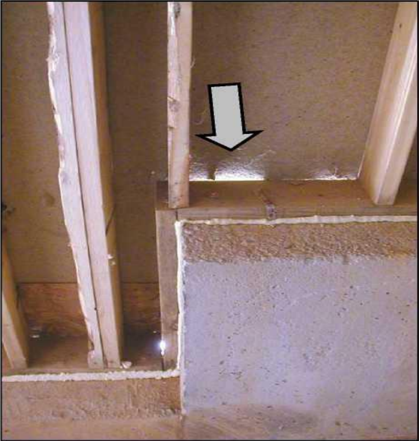
INCORRECT: Gaps in Sheathing
